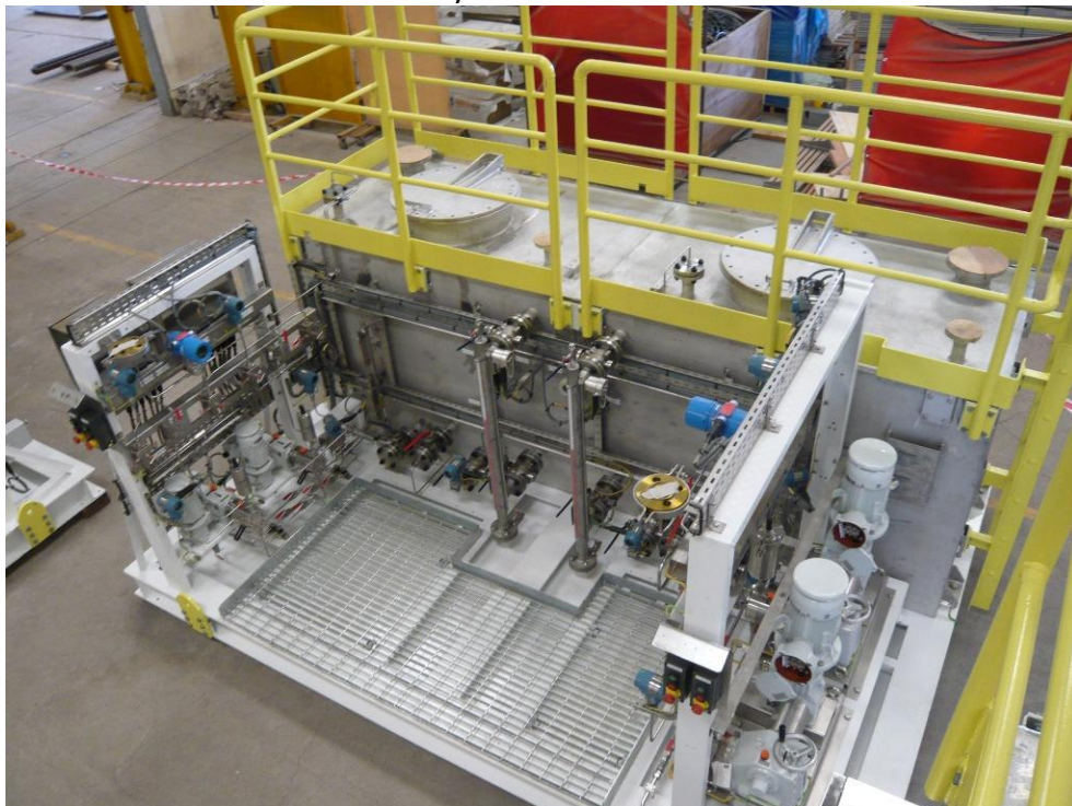
Methanol & Corrosion Unit
